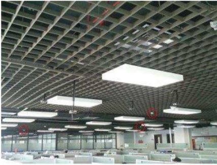
(c) Three-lamps, 9th floor, bldg. A
